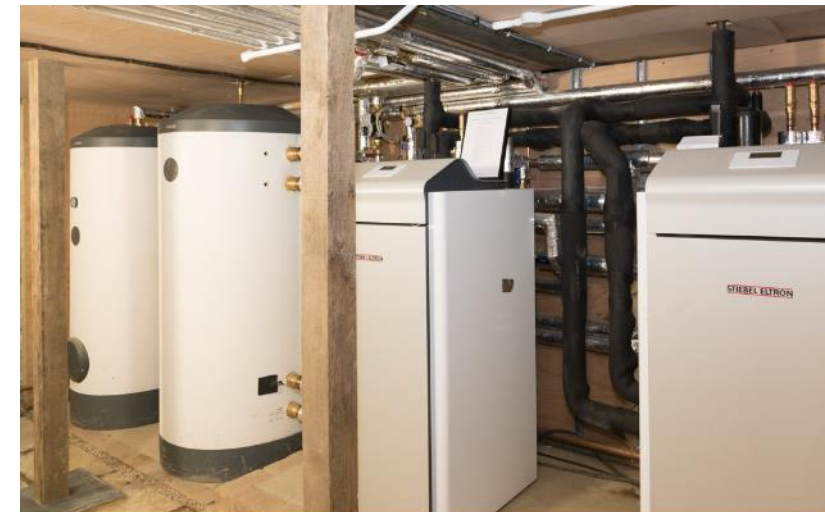
GSHP in Listed Farm House Sussex
