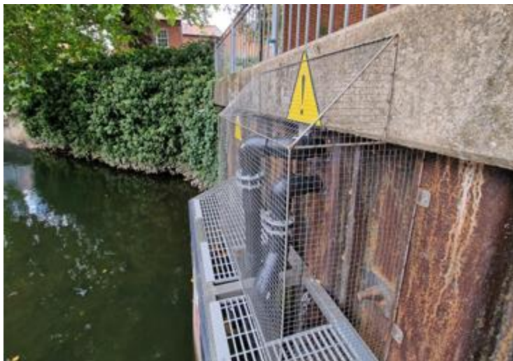
435kW ! Heat pump system for a social housing project with 86 houses
