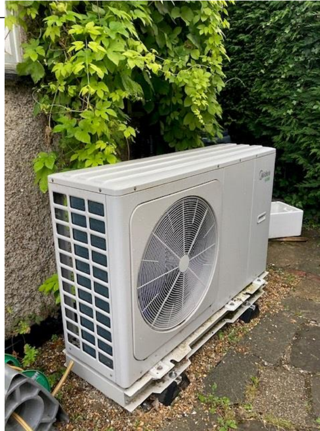
ASHP in house in Rodmell
